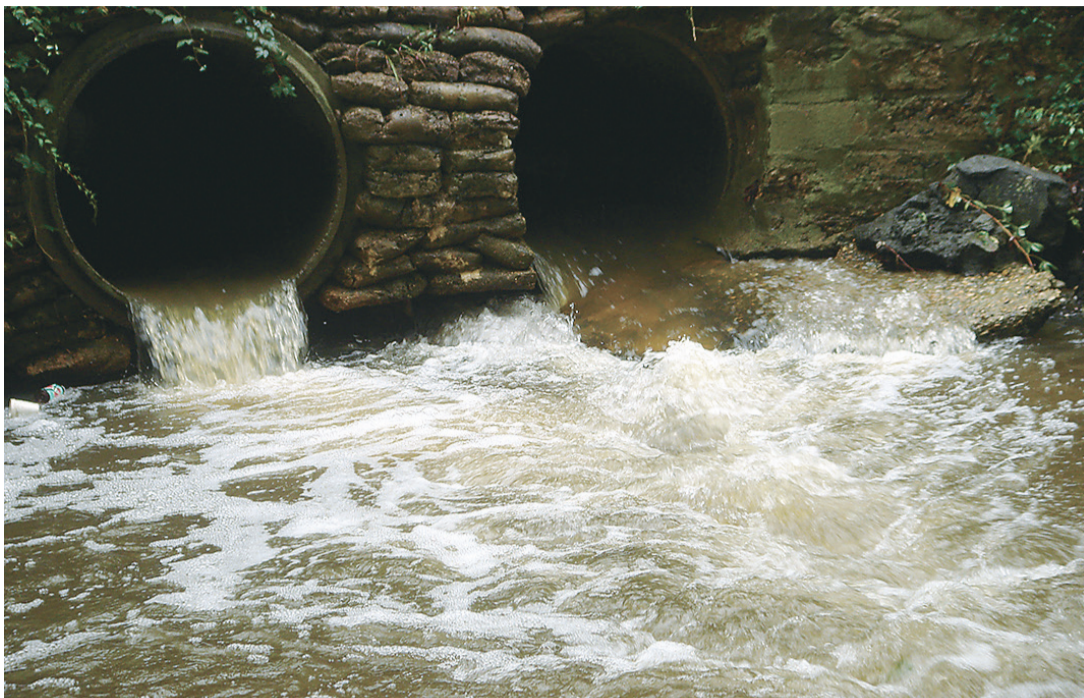
Stormwater flowing from an outfall in Paul Spring Creek in the Mount Vernon area during a storm.
